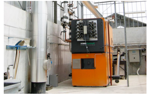
1'600 kilowatts wood heating system in a greenhouse at BioLand Agrarprodukte in Steinmaur ZH. Photo: Daniel Meier
