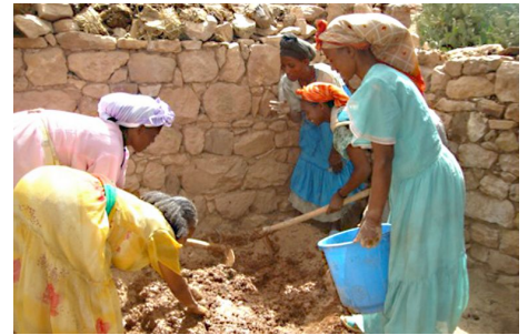
The efficient mogogo ovens are constructed by the village's women themselves.
