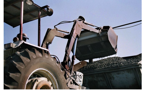
Prior to the project, the citrus processor in Limpopo consumed coal to dry orange peels, releasing climate-damaging emissions.
